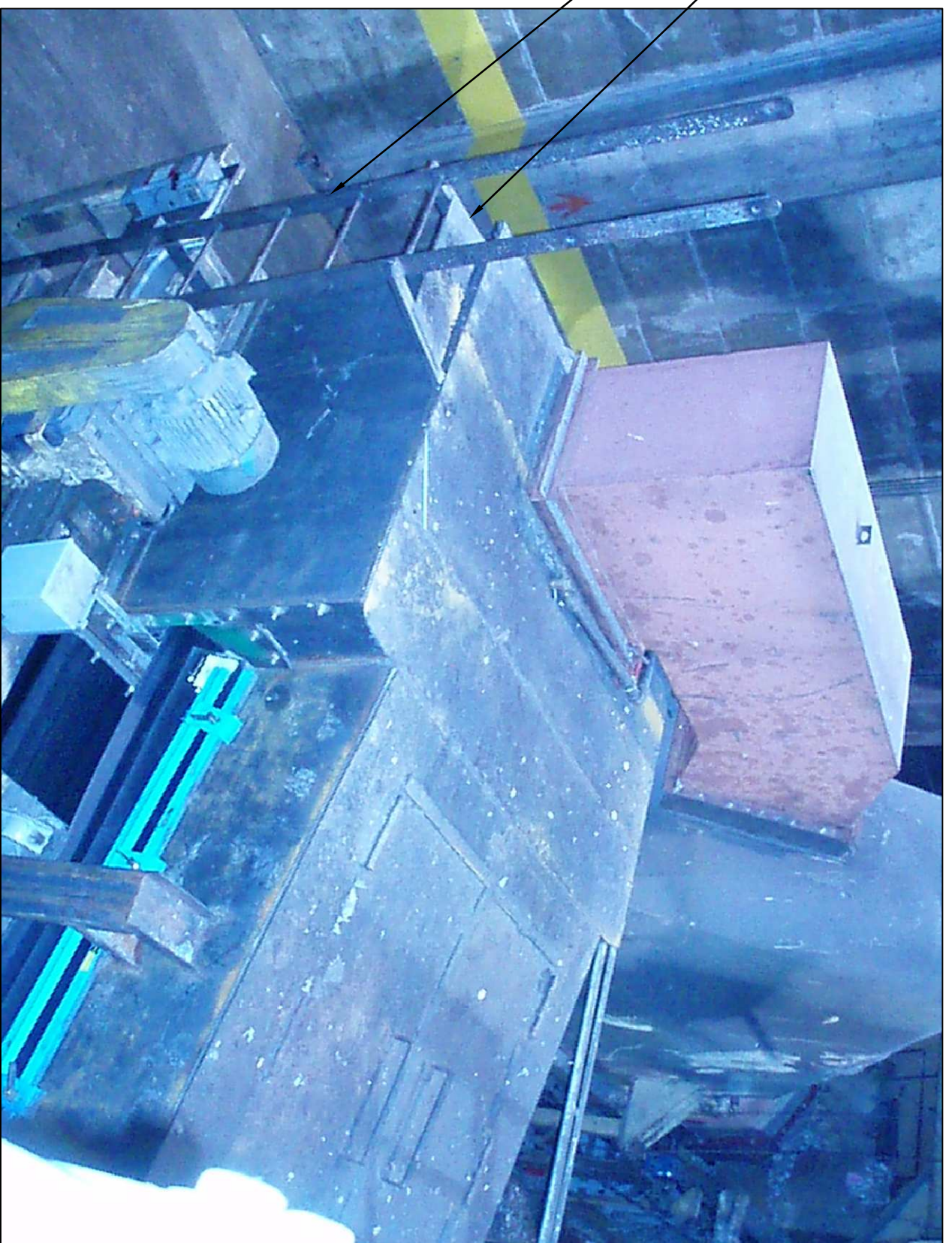
PICTURE OF EXISTING SECONDARY SHREDDER DISC. CONV. 133 (NTS) (LOOKING NORTH-EAST)
