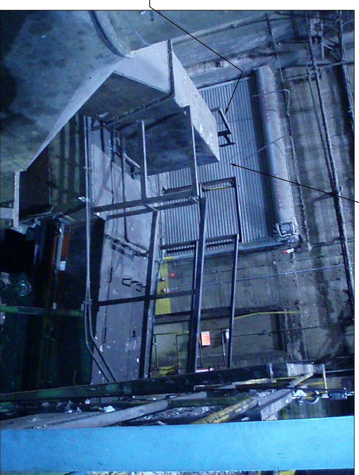
PICTURE OF EXISTING GUARDRAILS AT SECONDARY SHREDDER DISC. CONV. 233 (NO SCALE) (LOOKING NORTH-EAST)
