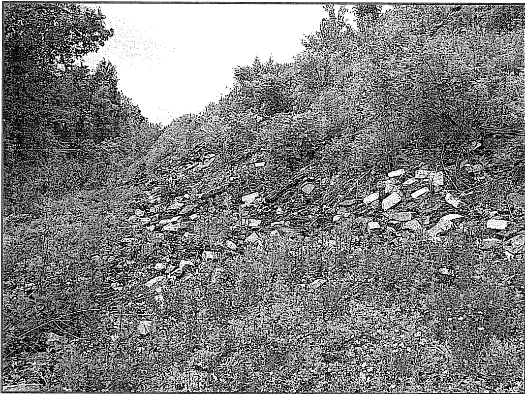
Photograph of the asphalt and urban fill earthen berm located on the southern and eastern portions of Area B on the site, facing west.
